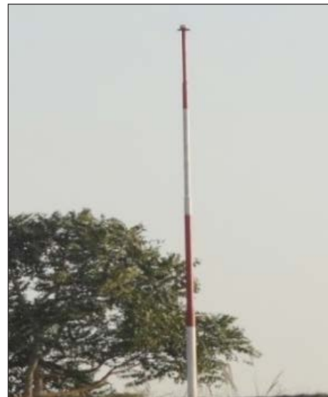
Light on Steel Pole
