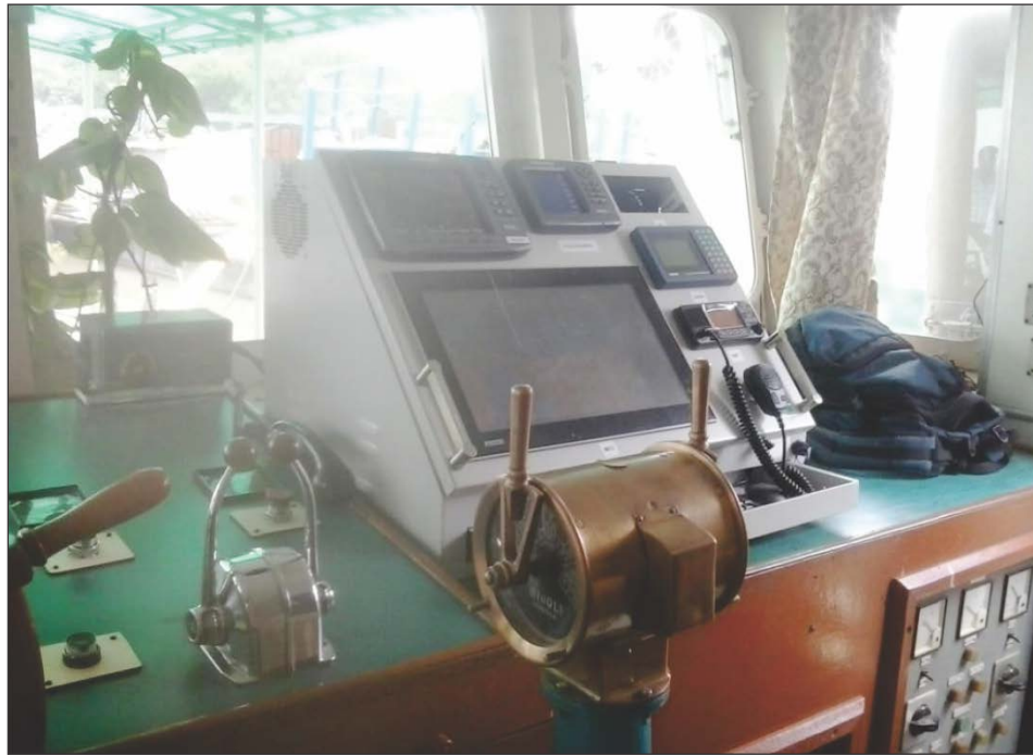
On board River Information system (RIS) equipment
