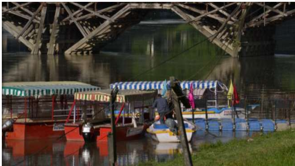
Figure 5-13 Picture Taken when the water transport was functional 2013
